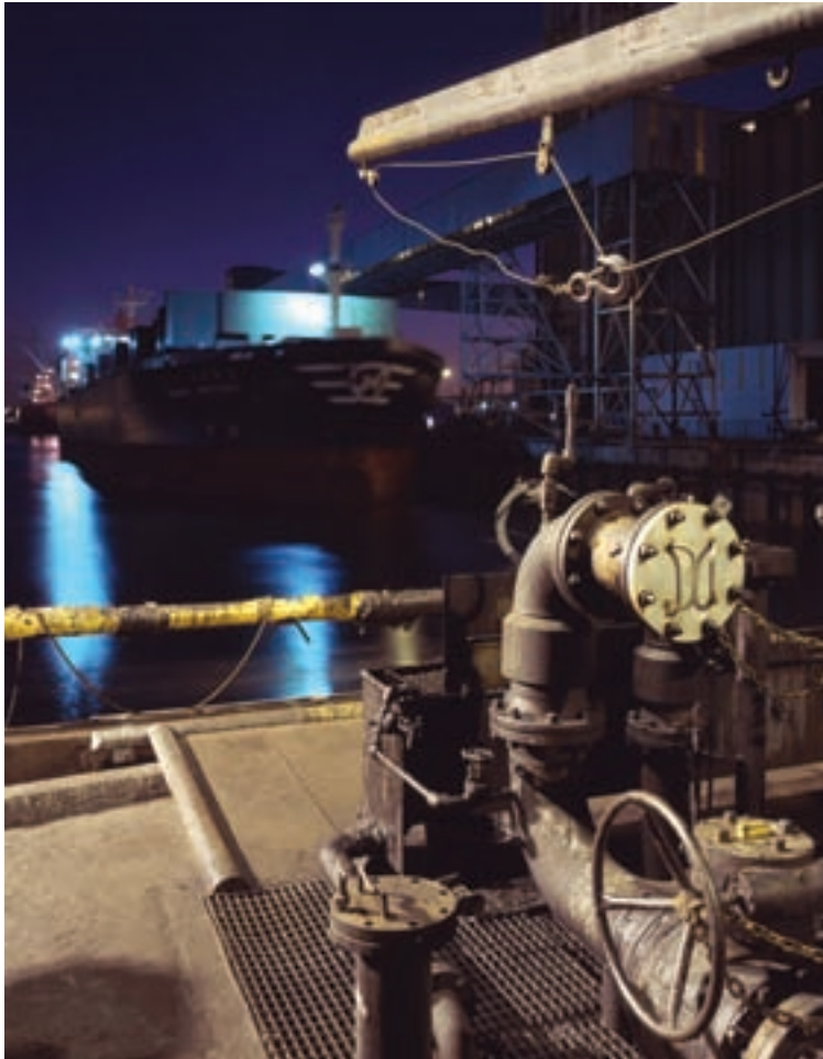
Oil Pumping Station; 5 minutes at f22, 120mm lens, Fuji 64T]
